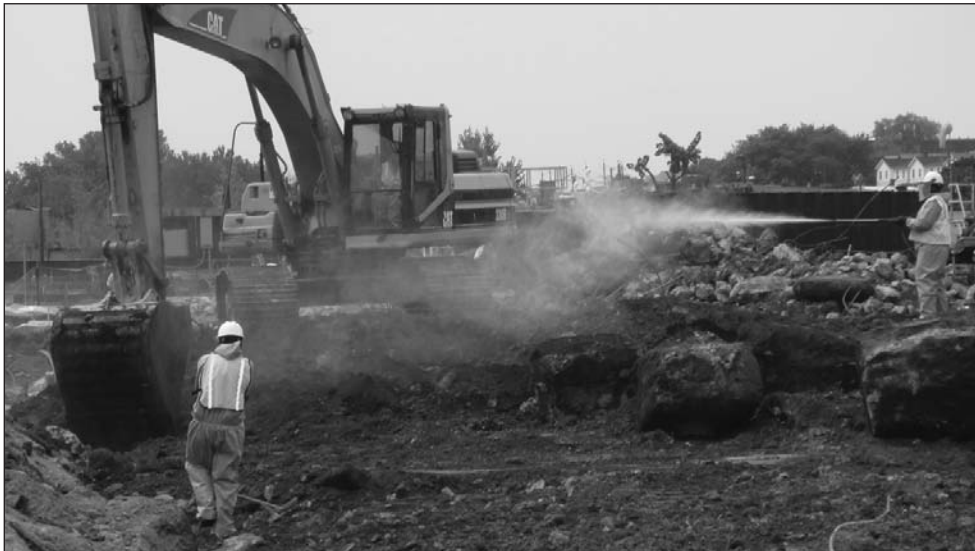
Excavation is the method of choice for cleaning up the Garfield Avenue Site, which PPG has been doing since July as part of the initial cleanup.
